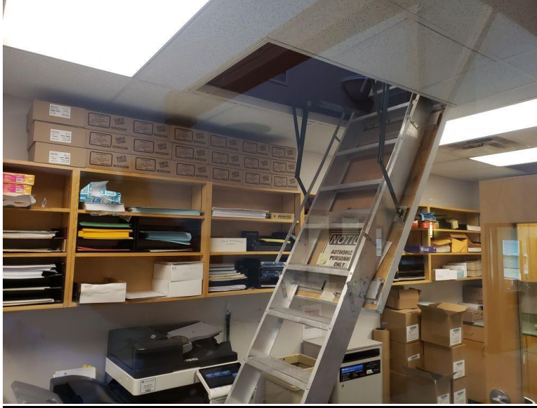
Stairs to Air Handler units.
